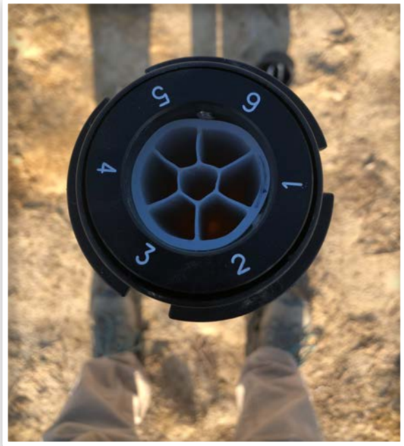
Top view of a CMT multilevel well. The multilevel has 7 depth discrete monitoring intervals.
